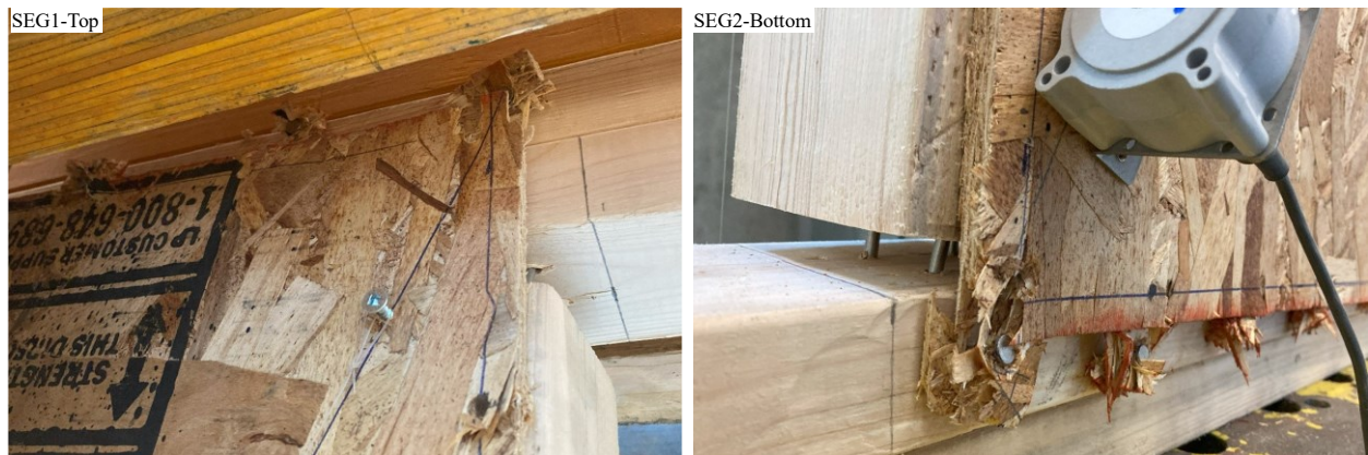
Figure 4.40: Nail failures at the top and bottom edges of the sheathing panel
