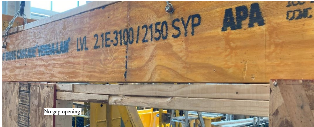
Figure 4.43: Formation of the gap between shear wall top plates and floor assembly.
