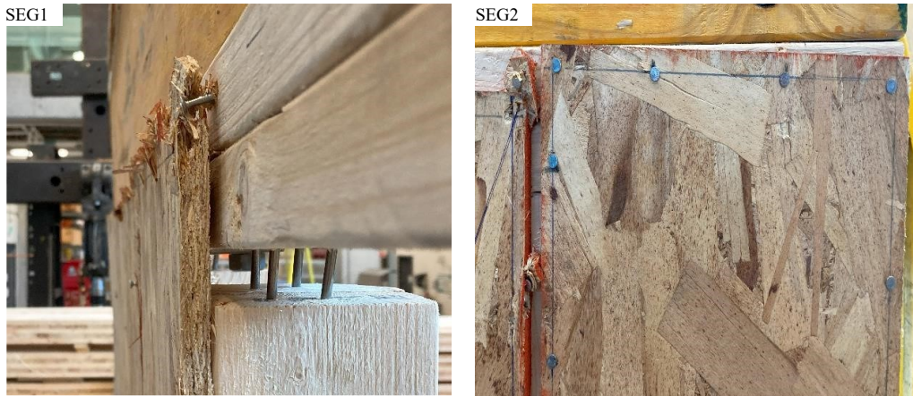
Figure 4.38: Top plates separation and nail damages at the top of shear walls (Configuration #3)
