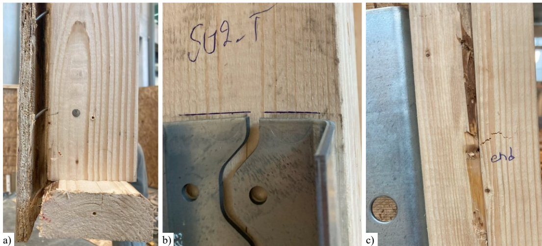
Figure 4.49: Failure modes: (a) nail failure and panel separation; (b) HD slippage; (c) chord fracture
