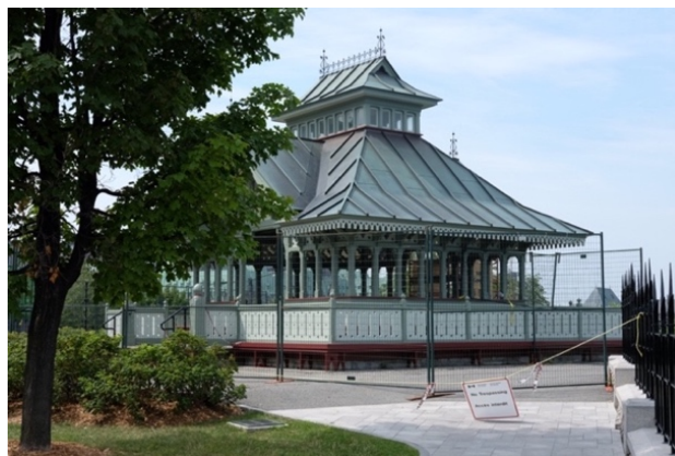
Figure 7: The Police Memorial Pavilion with a “No Trespassing” sign restricting public access for what seemed to be repairs (photo by Matthew Ferguson)
