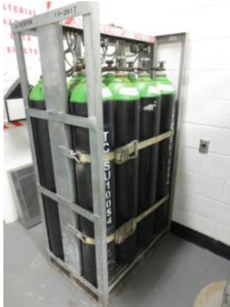
Figure 38. Propellant gas Bottle Pack. Consists of 11 Single Bottles. This Gas is Fed to the Pressure and Temperature Controller
