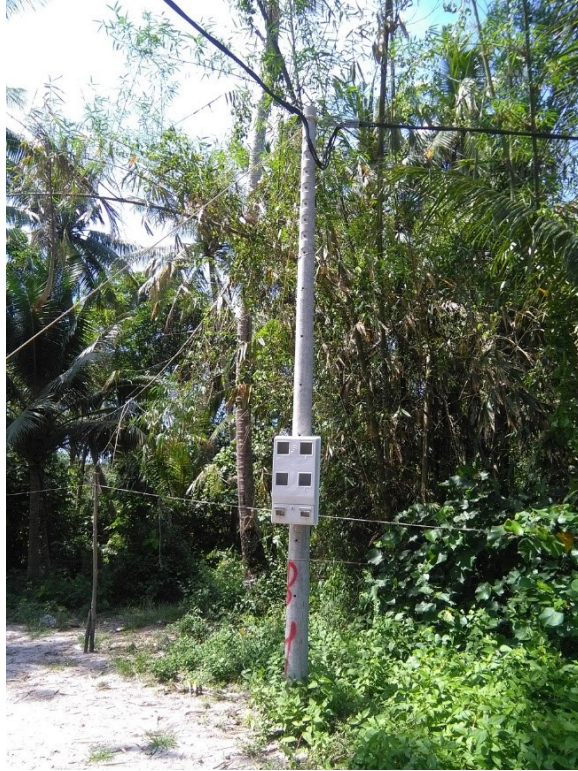
Figure 19. A newly installed utility poll for providing electricity in Koh Sralao. Photo taken in March 2017 by author.
