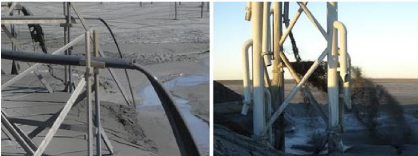
Figure 2.13. Thickened tailings discharge at Kidd Creek, ON, Canada (left) and at Mt. Keith, Western Australia (right) (Engels, 2002)
