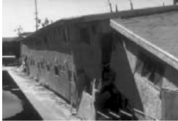
Figure 1.2: Meadows Apartment Complex, 1994 Northridge Earthquake (Lam et. al 2002)
