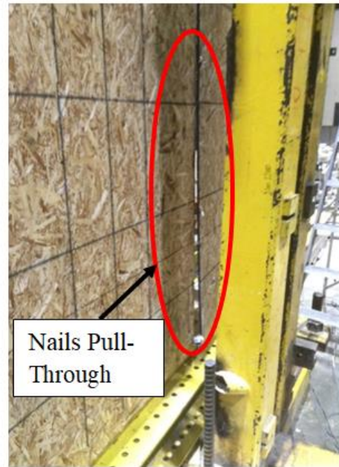
b) SW-2E (One 2"x6" End Stud) Nails Pull-Through Where Two Panels Join
