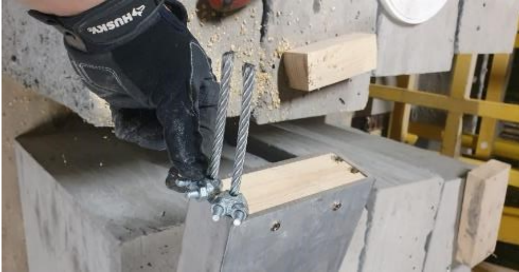
Figure 3.4: Wires anchored to the mullion (bottom of the mullion)
