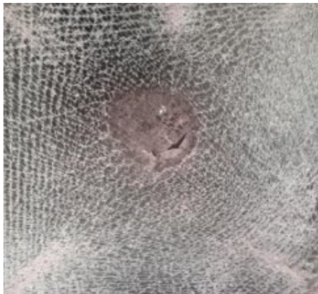
Figure 2.28: Failure of glass pane (with protected film) (Alameer, A., 2020)
