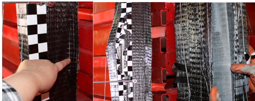
Stages of CFRP debonding
