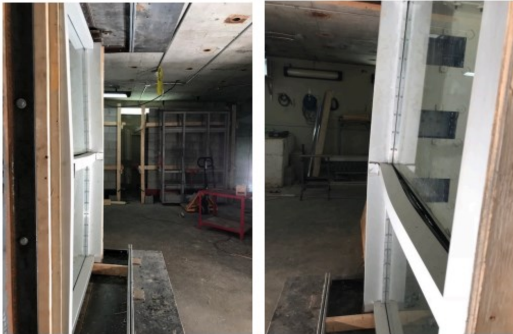
Figure 2.43: Performance of curtain wall during Test 3 (Saatcioglu et al., 2017b)
