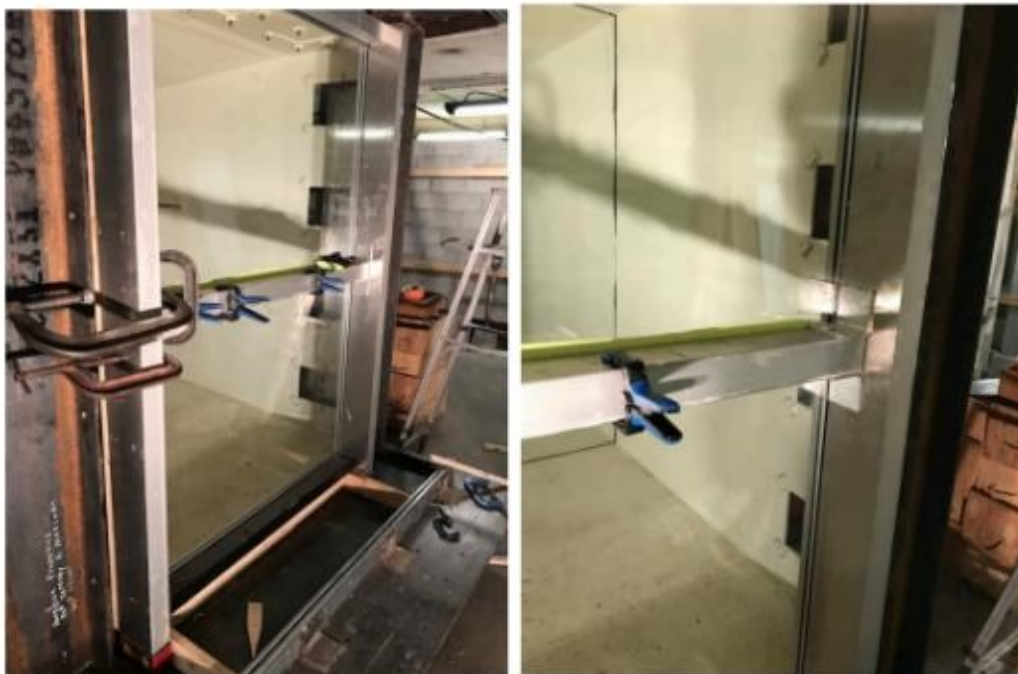
Figure 2.44: Application of aluminum plates and angles with epoxy adhesive for strength enhancement (Saatcioglu et al., 2017b)
