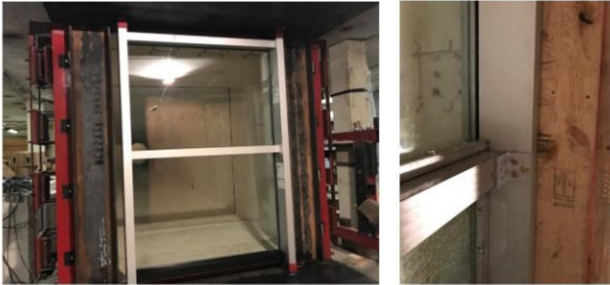
Figure 2.37: Curtain wall 2 prior retrofitting (left) and Curtain wall 2 after retrofitting (right) (Saatcioglu et al., 2017a)
