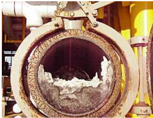
Figure 1.10: Pipeline plug due to formation of methane hydrates. 60
