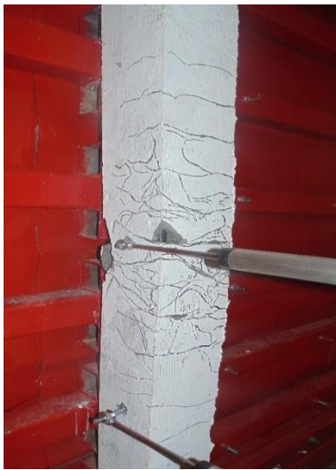
e) Tension face at blast 3
