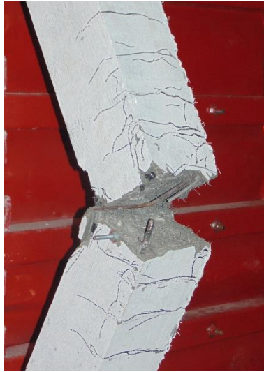
f) Mid-span and bar rupture at blast 4
