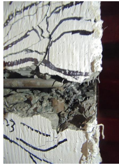
g) Bar rupture at blast 4
