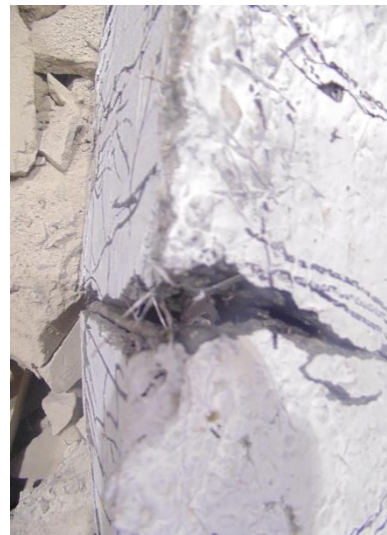
h) Bar rupture at blast 5
