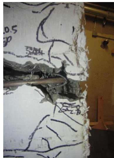
g) Bar rupture at blast 4
