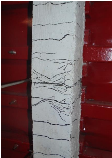
e) Tension face at blast 3
