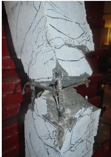
f) Mid-span bar rupture at blast 4
