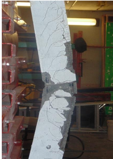
g) Mid-span at blast 5
