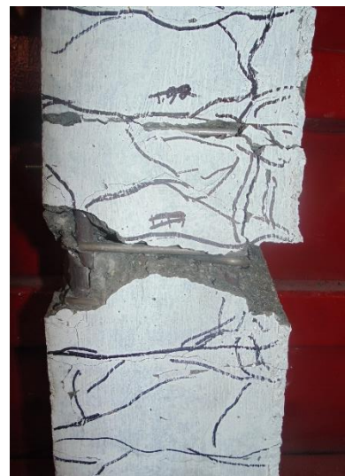
g) Bar rupture at blast 4
