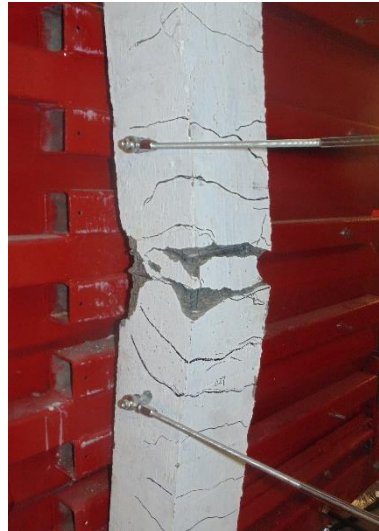
e) Tension Face at blast 3
