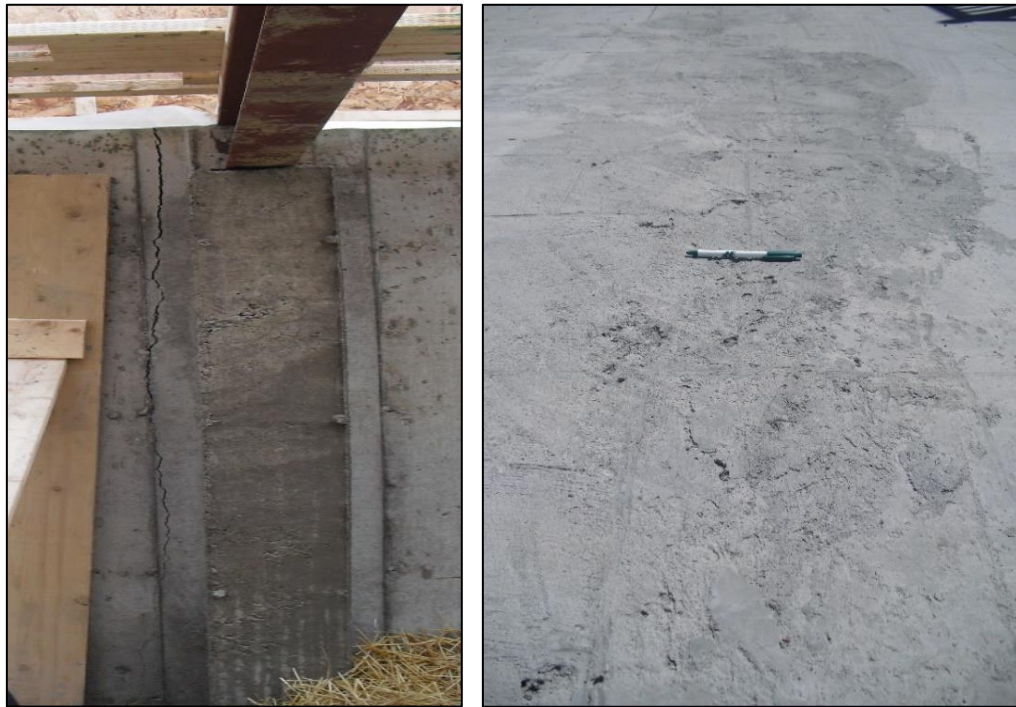
Figure 2-1: Incorrect concrete setting determination results in permanent cracking (left) and improper surface finishing (right)
