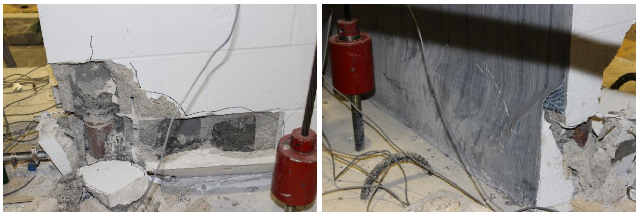
Figure 171.36 West side toe region of the wall at 2.25% drift
