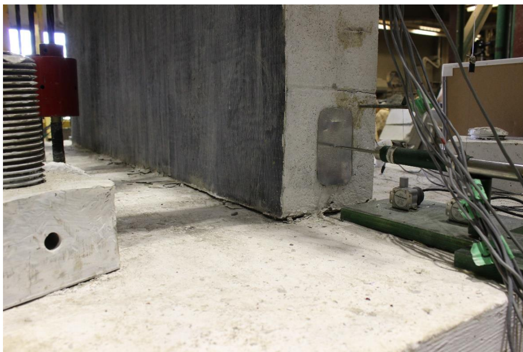
Figure 142.7 Wall 1 uplift of wall at west toe, 0.5% drift push
