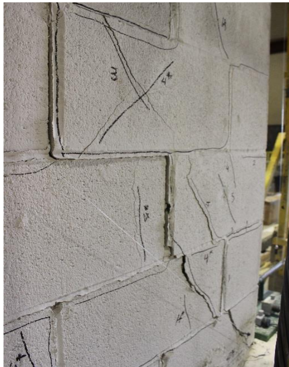
Figure 140.5 Out-of-plane movement of concrete blocks along the diagonal crack
