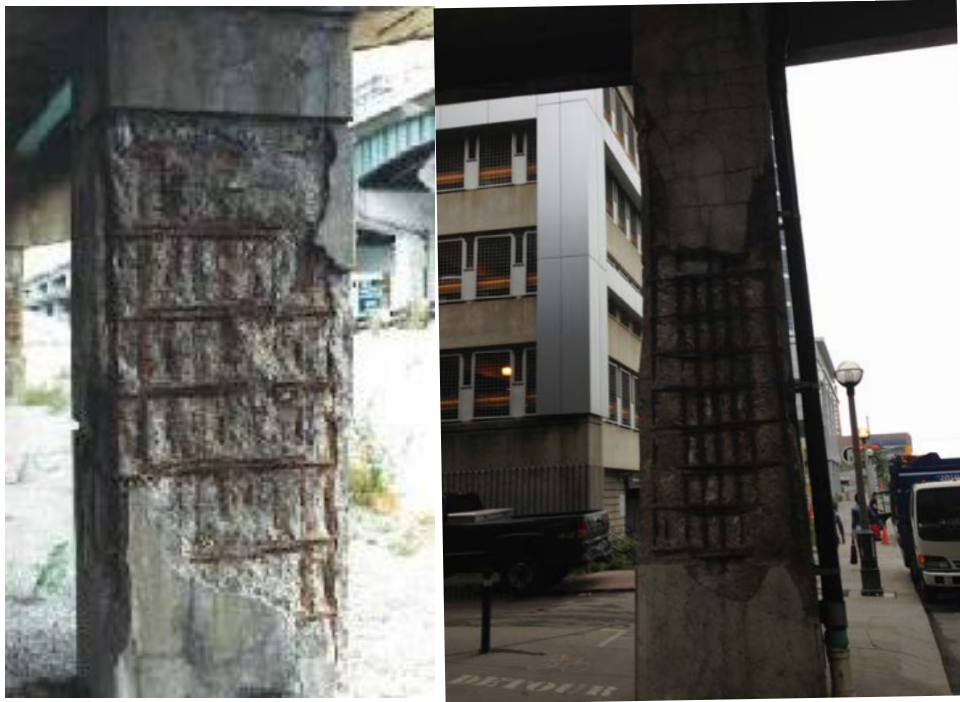
Figure 3.11-b-i: Case study V: sample slab-on-girder bridges with partial corrosion damage (Gardiner Parkway-Expy, Toronto, Canada).
