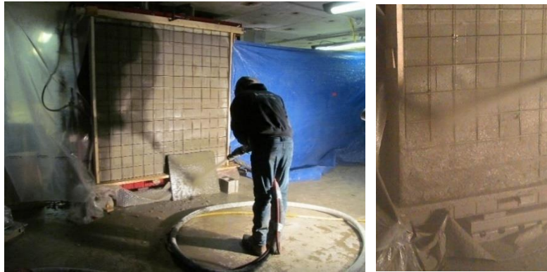
Figure 3-13. Nozzleman tests the consistency of the shotcrete before applying it to the wall
