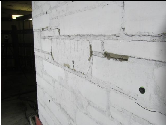
G) Shot 8 Failure
