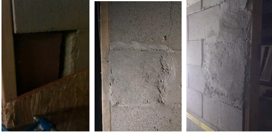
Figure 3-11. Damage and Repair of RMW-C-L
