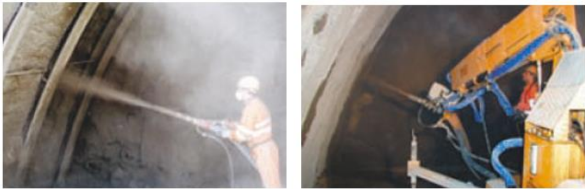
A) B) Figure 2-10. A) Dry spray and B) wet spray shotcrete (Hofler and Schlumpf, 2004)
