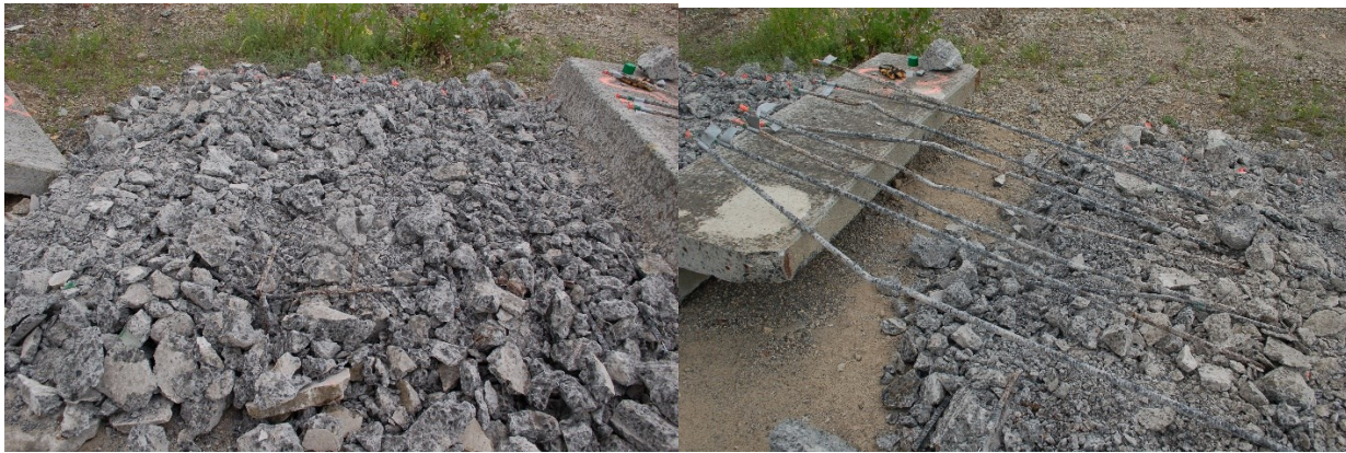
Figure B.0.6: Slab 13 Exposed Rebar / Removed Rebar
