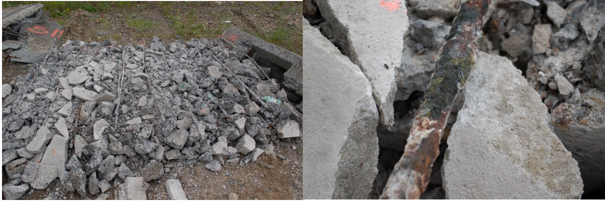
Figure B.0.5: Slab 12 Exposed Rebar / Evidence of Green Rust
