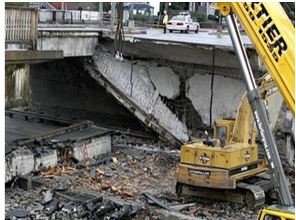
(b) The collapse of de La Concorde Bridge due to shear failure
