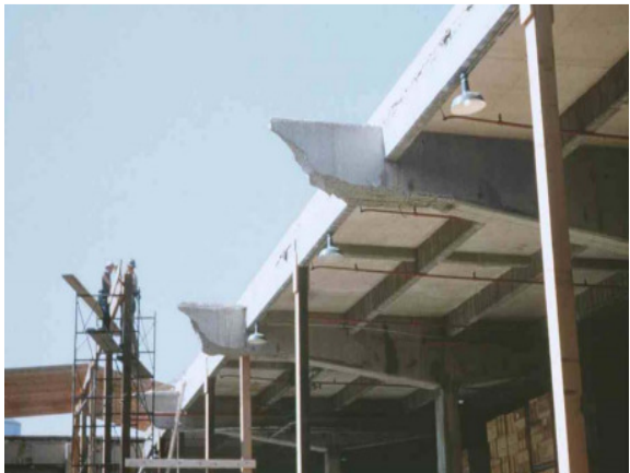
(a) Beams failed in shear at the US Air-force warehouses
