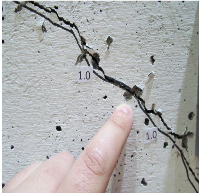
Figure 5.9: The influence of high-strength fibers on crack width
