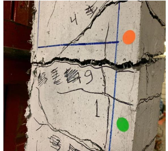
g) Mid-span fiber pullout (Blast 3a)
