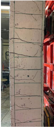
d) Mid-span cracking (Blast 2c)
