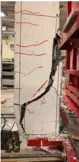
c) Shear failure (Blast 2a)
