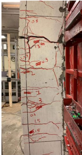
e) Mid-span concrete crushing (Blast 2c)
