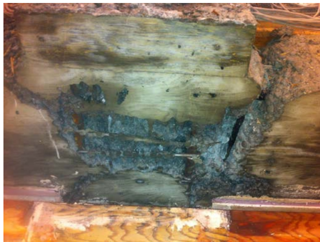
Figure 3.13 Poor consolidation of concrete in the plastic hinge region for first D/4-1.0% beam
