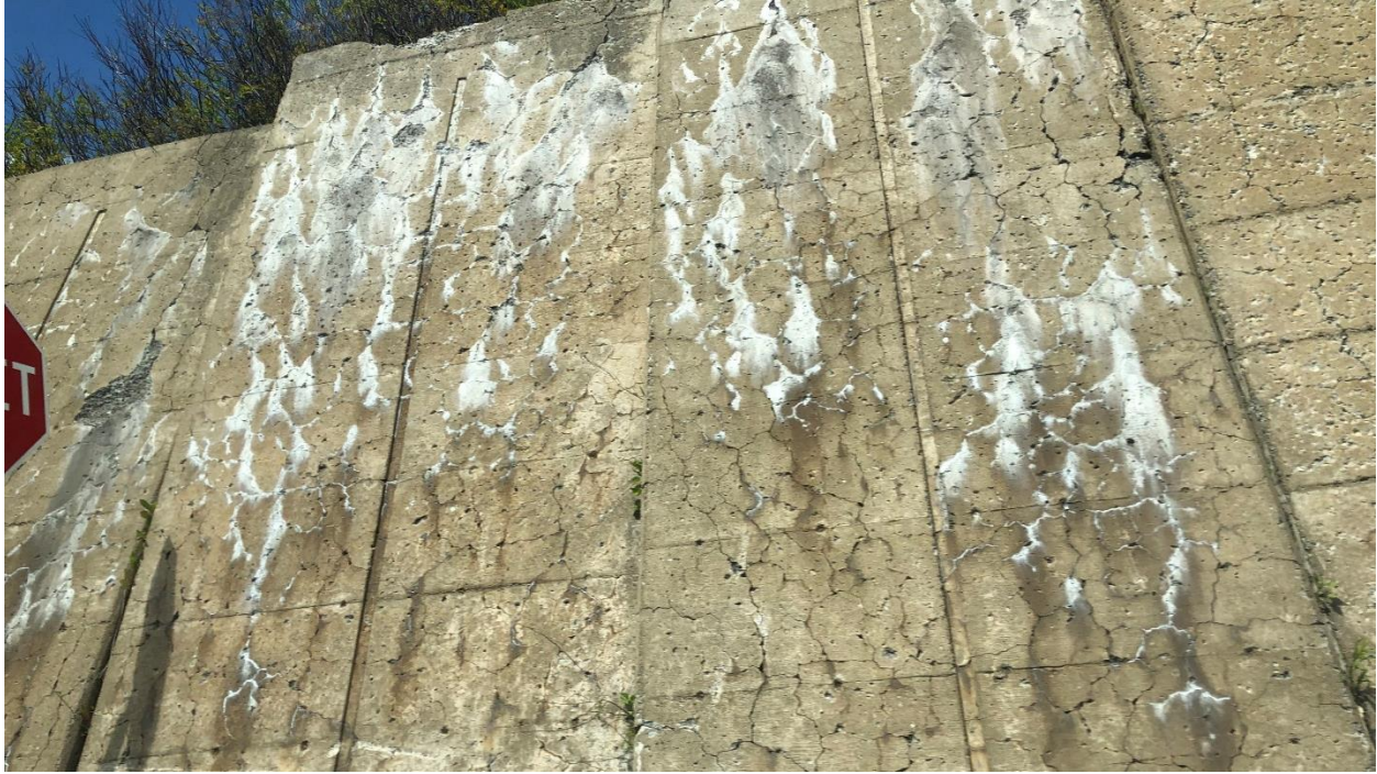
Figure 2.1. ASR-affected concrete retaining wall next to an on-ramp in Québec.
