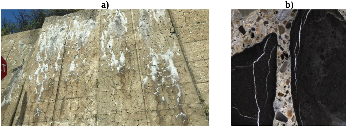
Figure 9.1 Likely ASR-affected concrete from a) a retaining wall next to an on-ramp in Québec City, Canada and b) a micrograph from a core of a nearby decommissioned overpass (Du Vallon-Charest, Québec) with a field of view of 1 cm by 1 cm where the white lines are cracks in the aggregates filled with reaction product.
