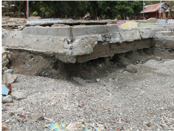
Figure 4-1. Scour under a coastal structure observed immediately following the 2018 Indonesia tsunami event in Palu Bay (courtesy of Jacob Stolle, 2018).
