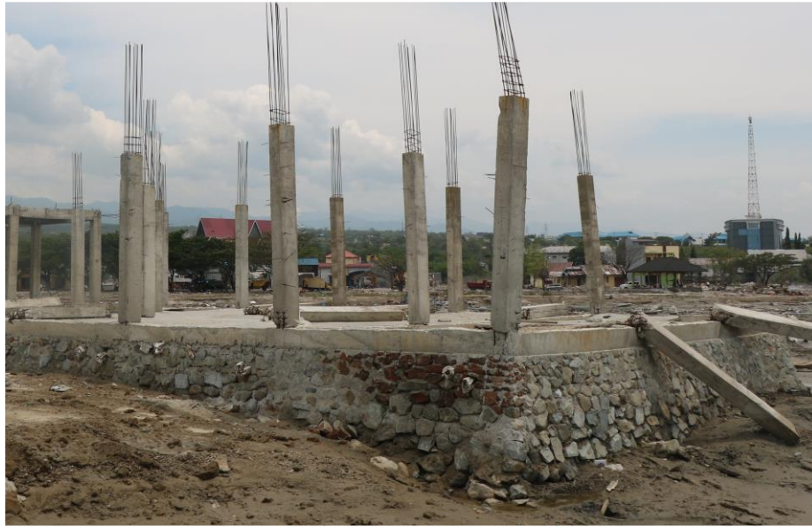
Figure 5-1. Image of extreme erosion around a foundation due to tsunami loading in Palu Bay, Indonesia (courtesy of Jacob Stolle, 2018).
