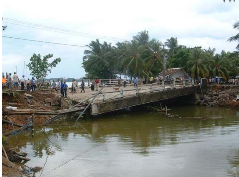
Figure 1-2. Collapsed bridge due to scour and erosion around its abutment (Rossetto et al., 2007)
