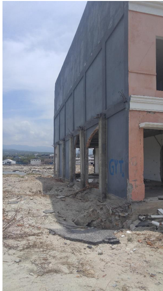
Figure 6-1: Image of local bed erosion around a residential building due to the 2018 Indonesia tsunami in Palu Bay. (Courtesy of Jacob Stolle, 2018).
