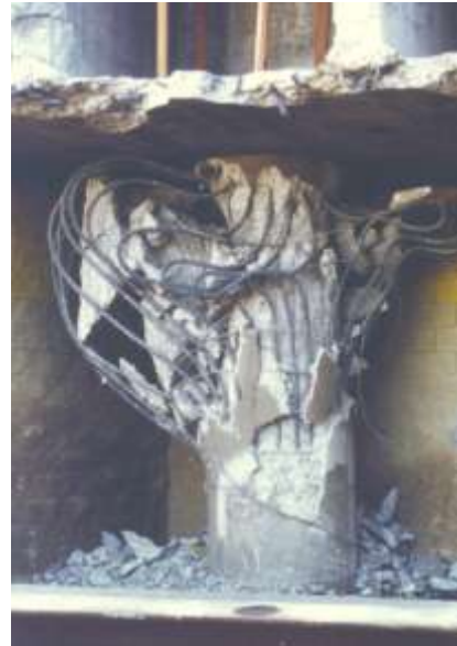
1994 Northridge Earthquake in California (Photo by Dr. Murat Saatcioglu)
