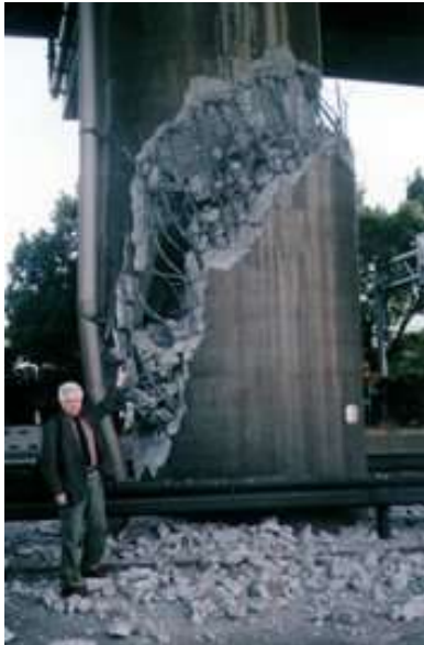
1995 Kobe Earthquake in Japan (Photo by Dr. Michel Bruneau)
