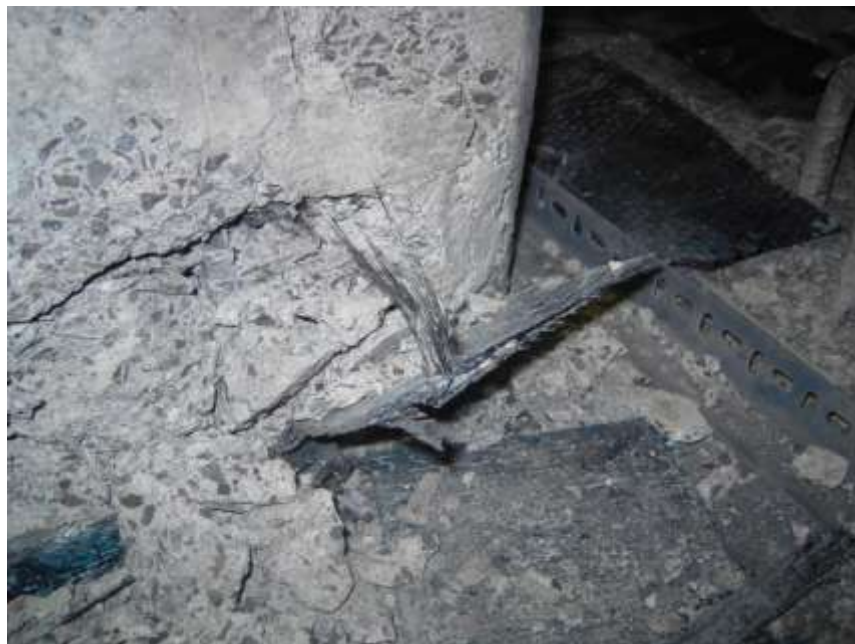
(f) Rupturing of cross-ties
