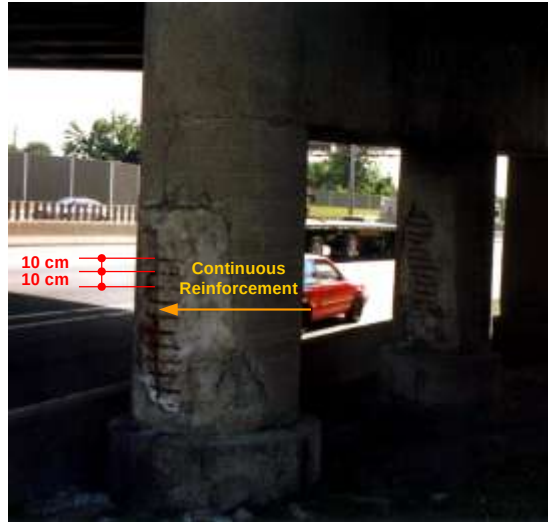
Fig. 1.10 Steel corrosion and spalling of cover concrete on a concrete bridge column
