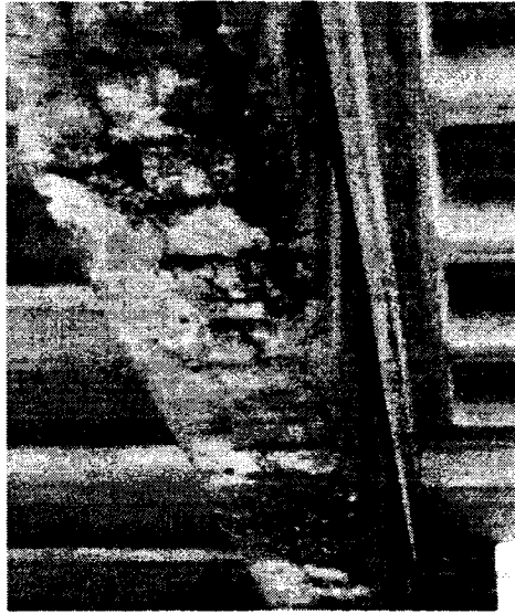
Fig. 1.1: Corrosion-induced damage in reinforced concrete
