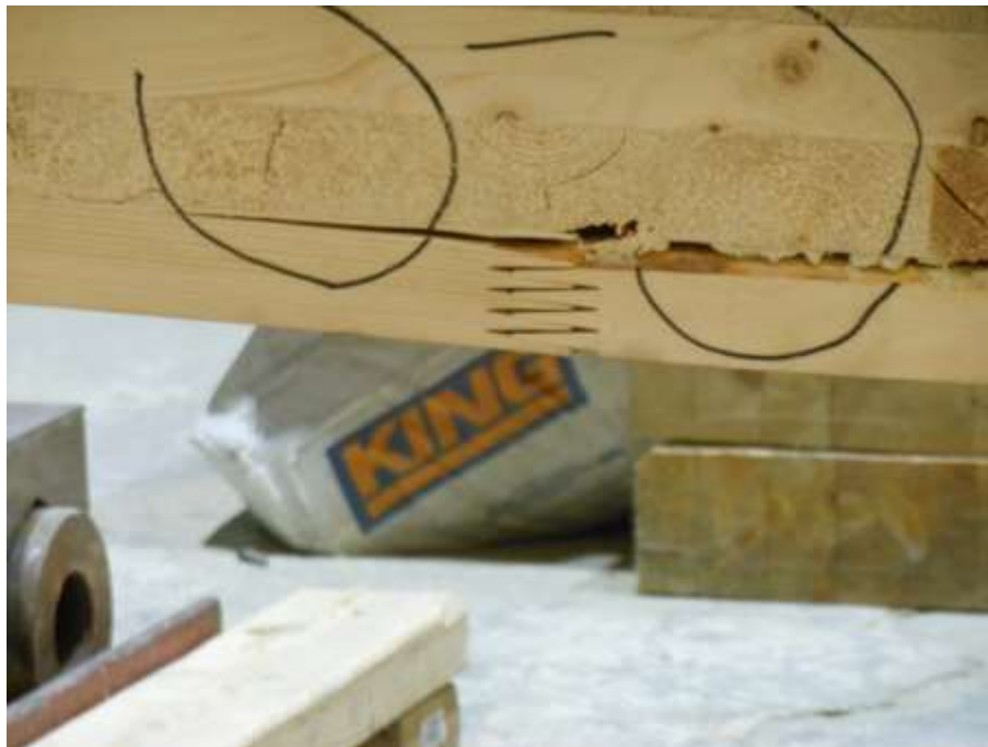
Figure A1.12: Separation of Finger Joints in CLT5-3
