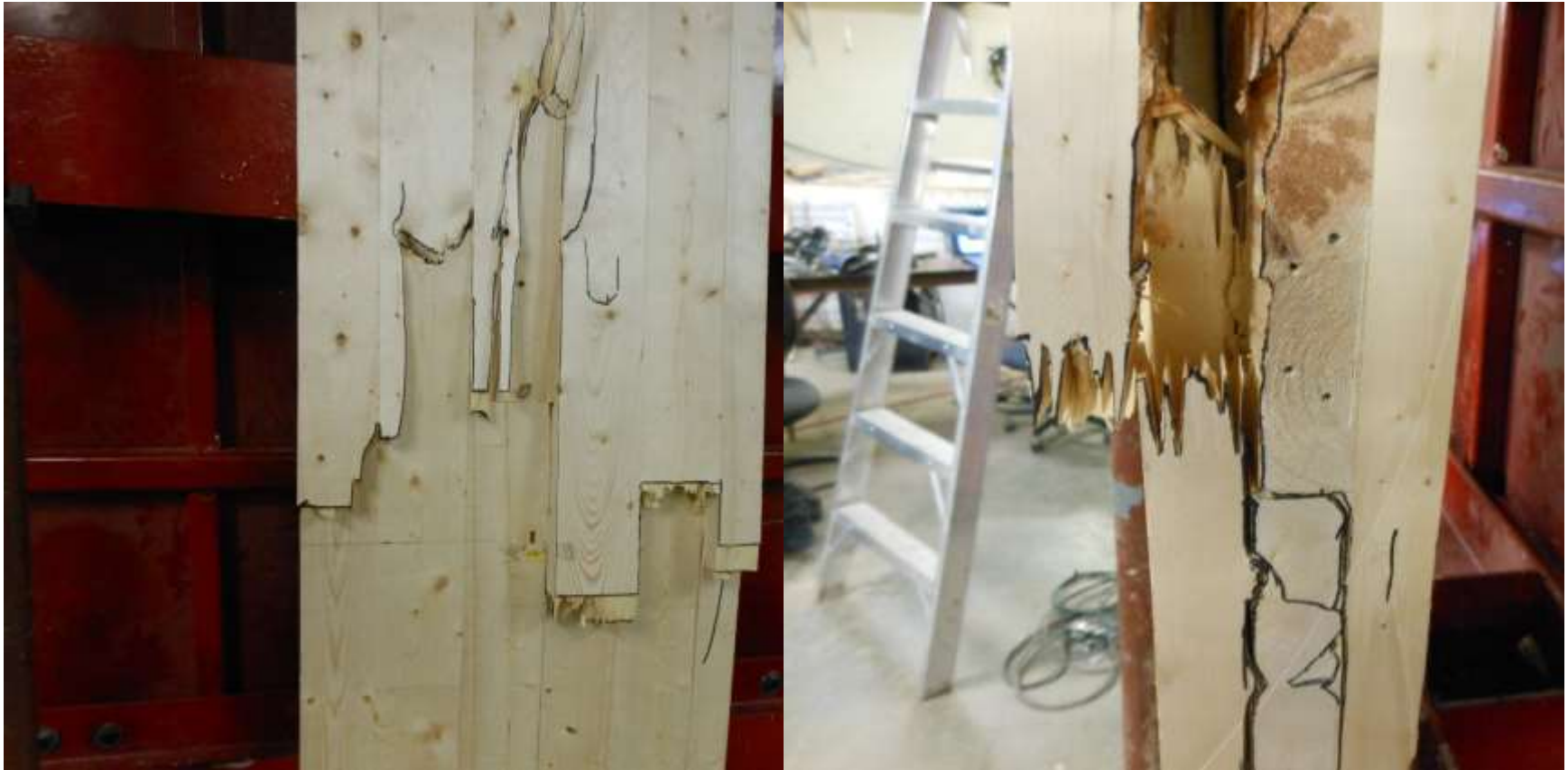
(a) Flexural Failure Along Finger Joints – Front Face
