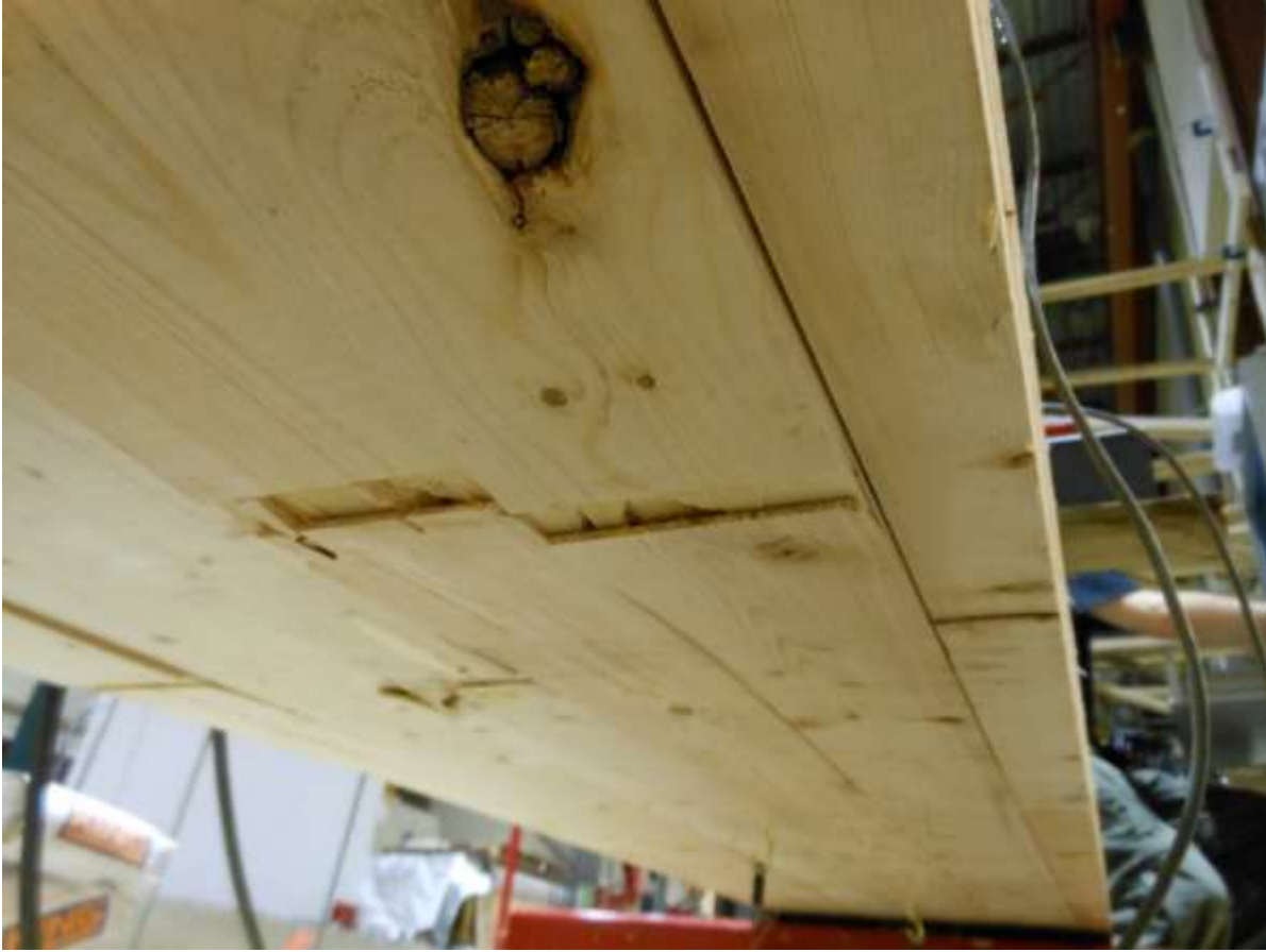
Figure 4.5: Multiple Finger Joints Separating in Tension Laminates of a 5-ply Specimen
