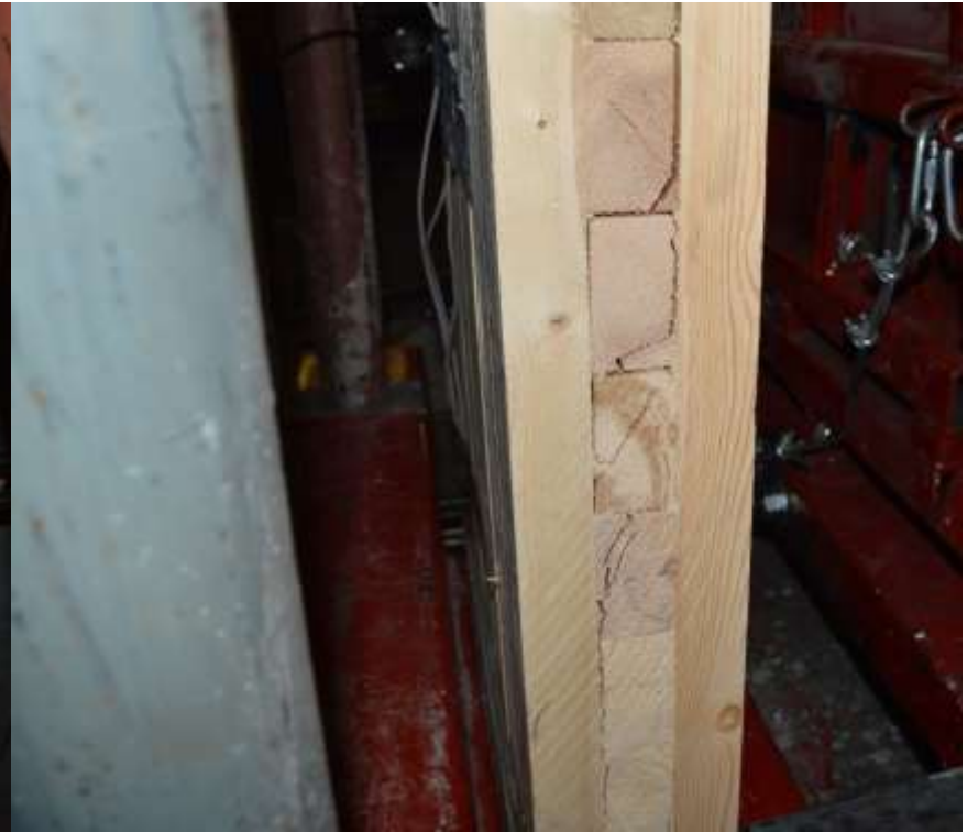
(b) Rolling Shear on Lower Right Side
