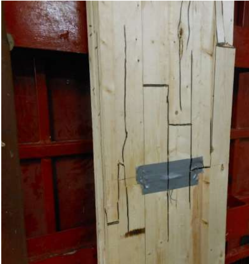
(a) Flexural Damage in Tension Laminates
