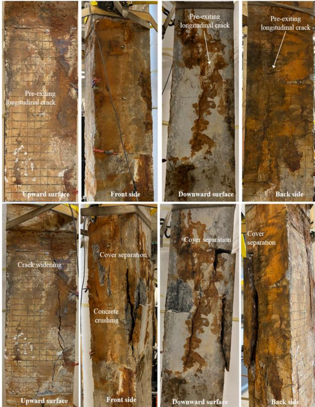
Fig. 4.10: Corrosion-induced damage before loading, Bottom: damage after loading (C-C-All)
