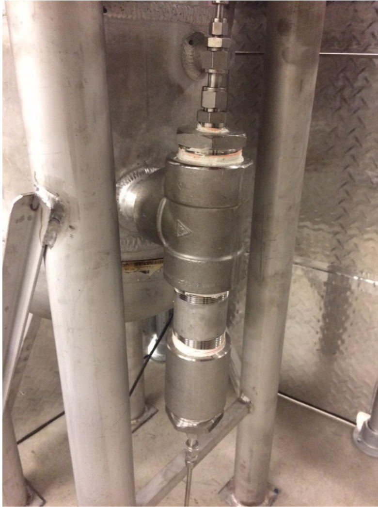
Figure A.3. Pressure vessel containing the feeder. Focus on the outlet tee used to discharge solids into the pneumatic convey line.
