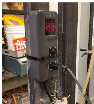
Figure Appendix 11-18: Programmable temperature controller for heating semi-continuous flow reactors.
