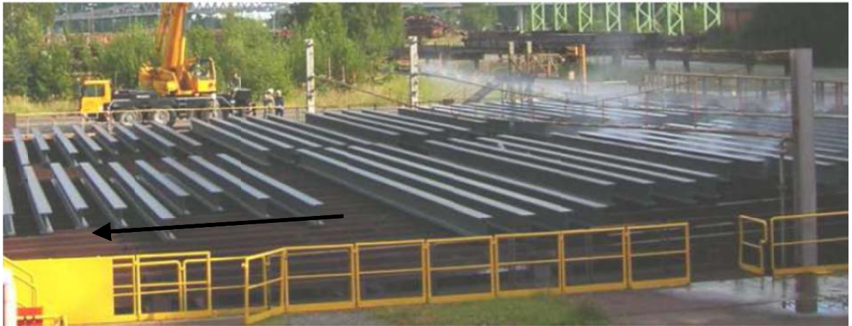
Fig. 1.6: A cooling bed for wide flange sections (Photo from Espinoza 2007)
