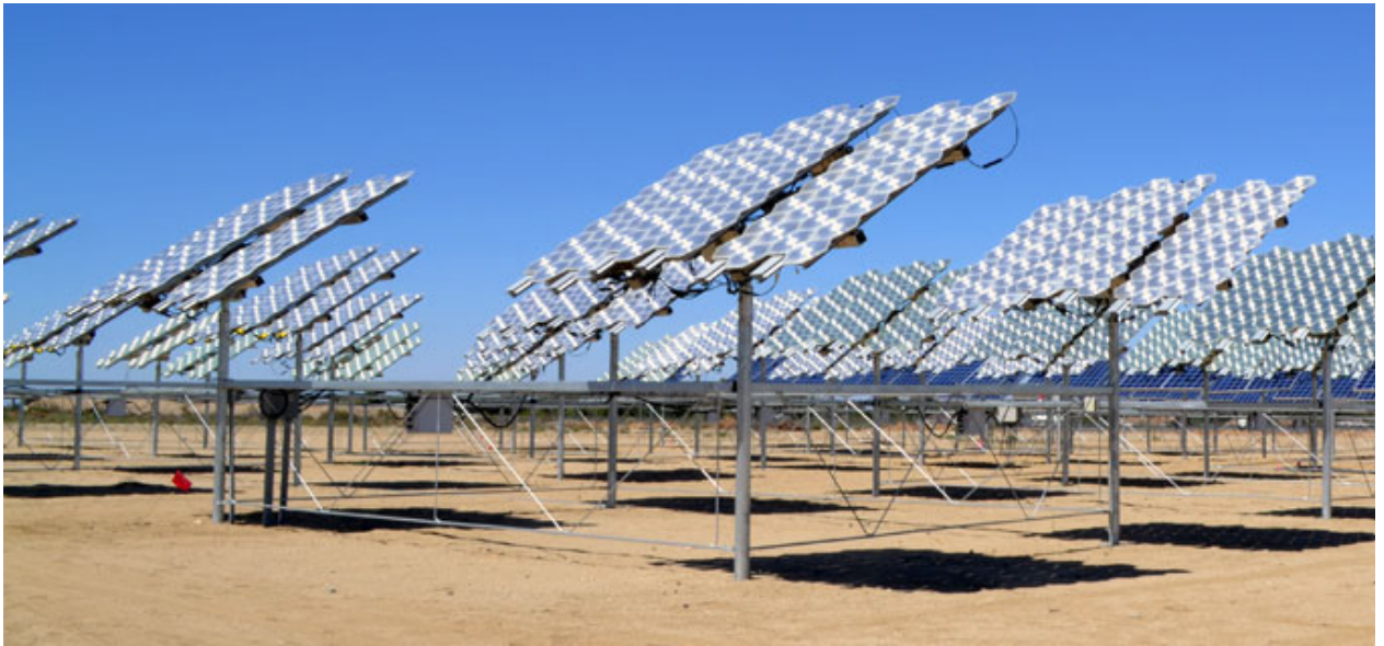
Figure 1.3: Morgan Solar’s Sun Simba CPV modules mounted on the Savanna trackers [5]. Four panels are mounted on each corner of the boxframe, which constitutes a single unit (cell) within a solar farm.
