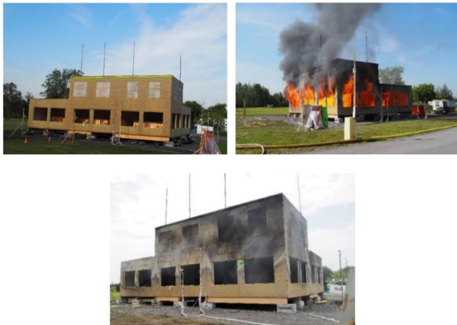
Figure 2-10 Full-scale mass timber structure used in Ottawa Fire Test: Before, during and after the fire test (Su et al., 2023).
