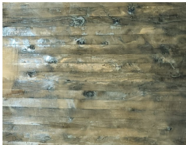
Figure 4-1 An example of the small fine cracks on the surface after char removal
