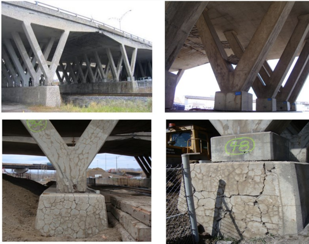
Figure 2.7: Robert-Bourassa/Charest (RBC) overpass affected by ASR in 50 years of service [3].
