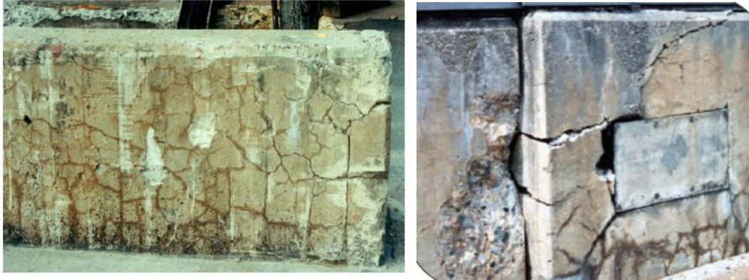
Figure 2.5: Typical ASR damaged concrete element with presence of spalling, deformation, joint closing, map cracking with the presence of gel product [3].
