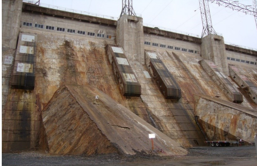
Figure 2.6 : Mactaquac Dam in New Brunswick, Canada affected by ASR [24].
