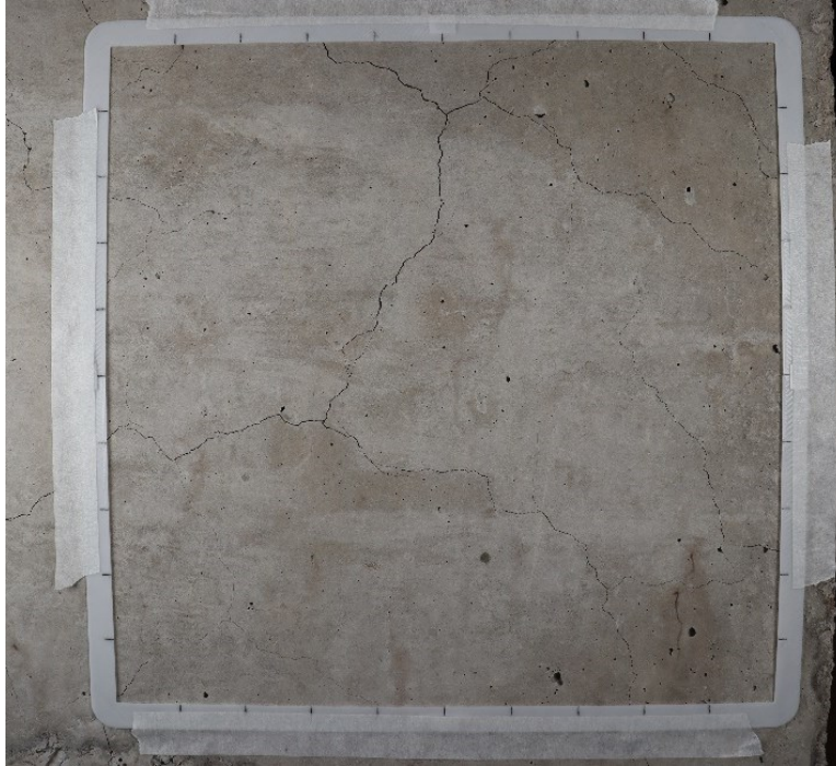
Figure 2.8: A typical cracking index layout on a concrete surface using a 3D-printed reference grid.
