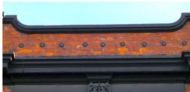
Figure 2-8: Example of through ties connecting the roof diaphragm to load-bearing wall (Ingham and Griffith, 2011a)
