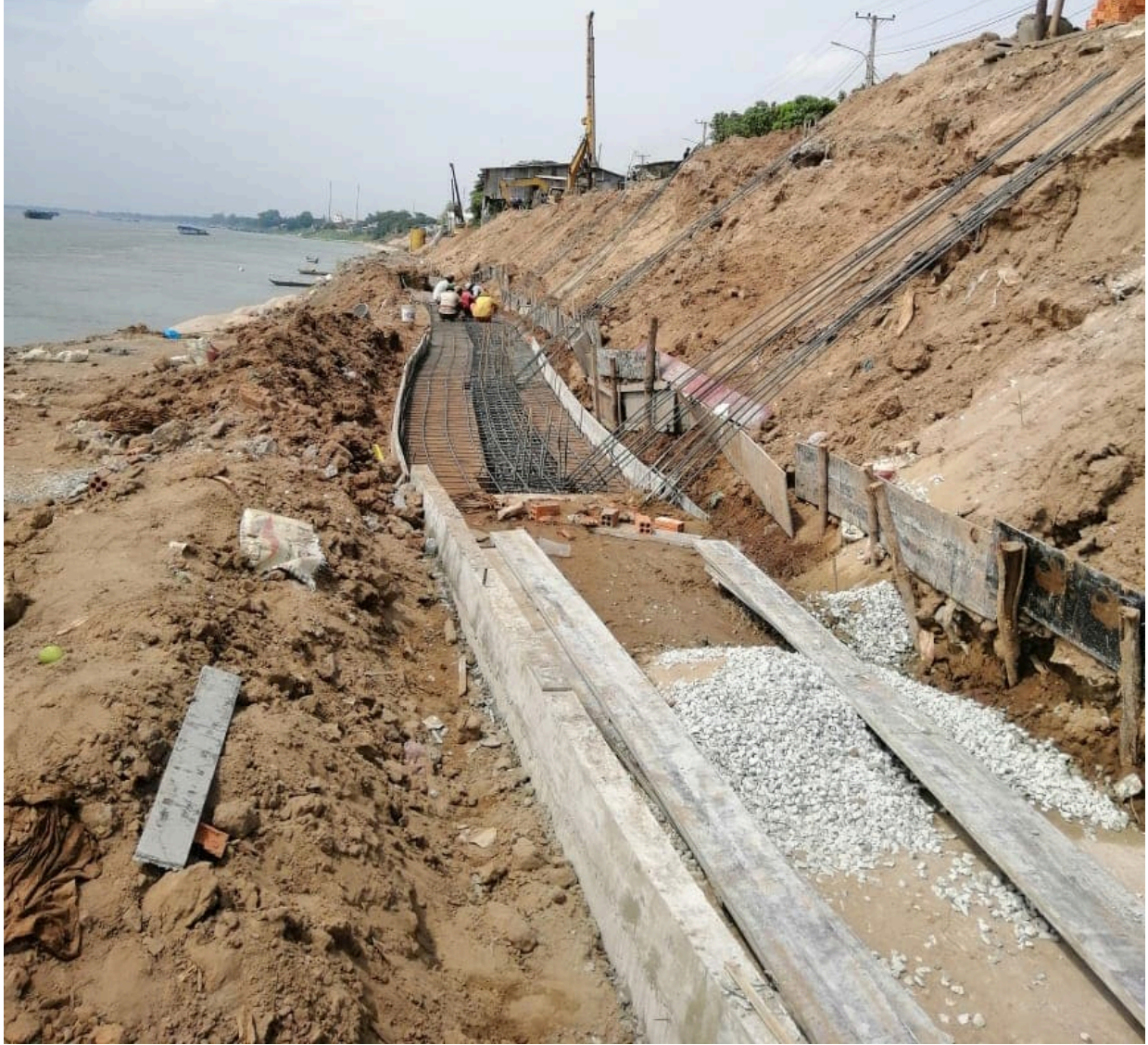
Figure 6.12 Concrete layer being constructed to reinforce a riverbank on the Mekong River.
