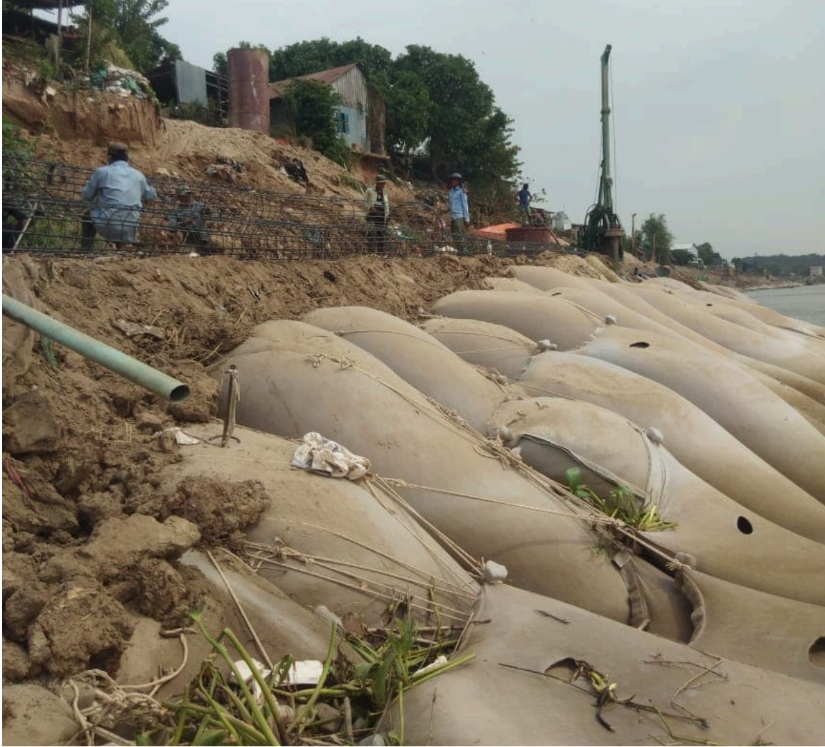
Figure 6.13 Sandbags used as structural reinforcement on eroding riverbank.
