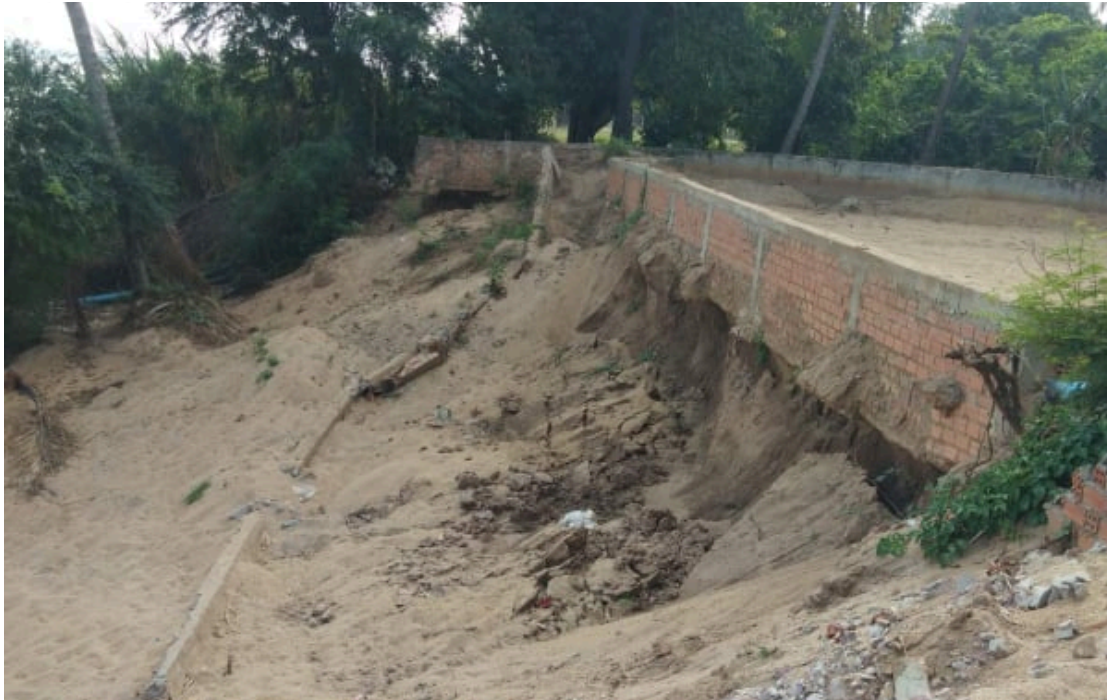
Figure 6.9 Erosion under a demolished house, on the riverbanks of the Mekong.
