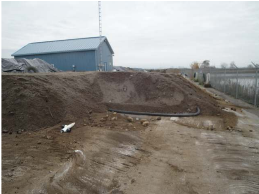
Photo B.4 Aeration piping system for biopiles
