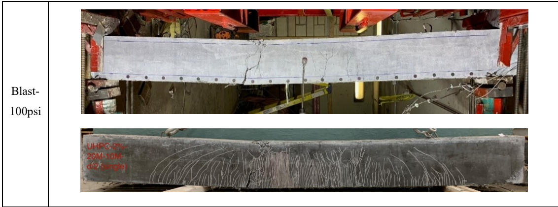
Figure A.105 Blast damage for beam U2-20M-DR-d/2
