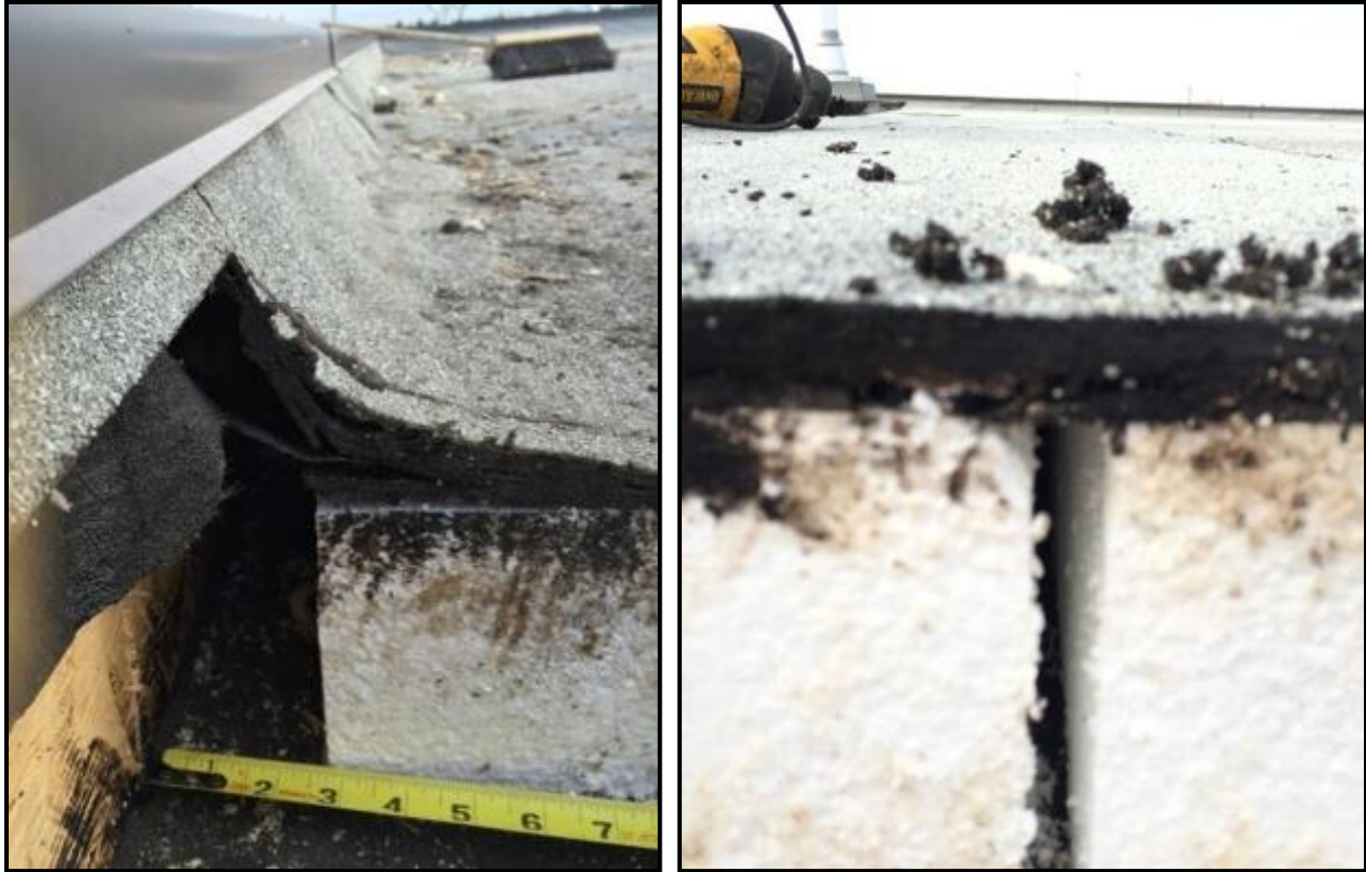
Figure 2-22: In-situ Insulation Gaps #2 (retrieved from the Canadian Roofing Contractors Association, 2016)
