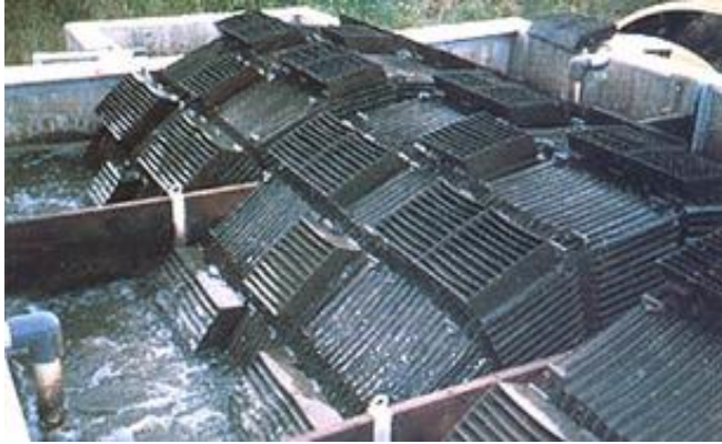
Figure 2.4 Rotating biological contactor (Triveni Engineering and Industries limited, 2013)
