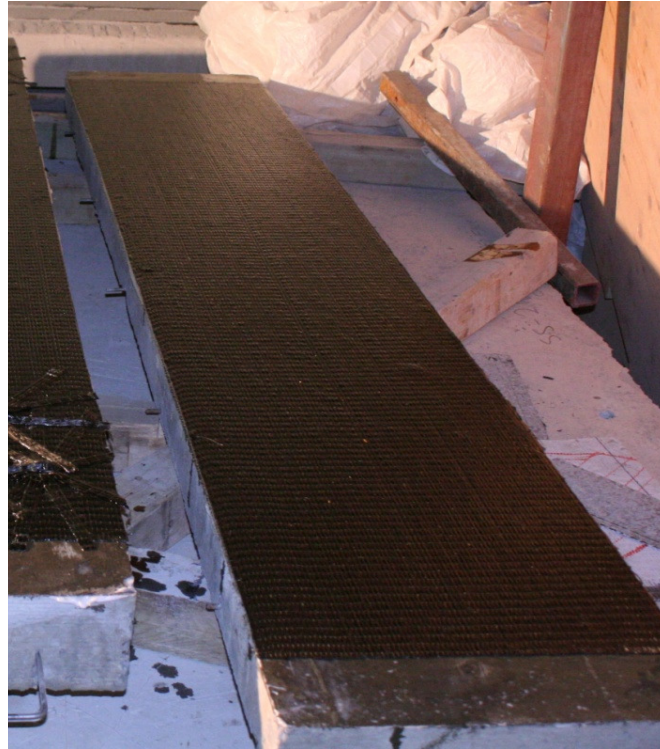
Figure 3.21: Typical One-way Reinforced Concrete Panel with Externally Bonded CFRP Retrofit Prior to Testing.
