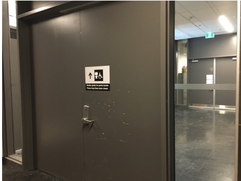
Figure 5-9 - STEM 3rd floor blocked path to "universally accessible" washroom
