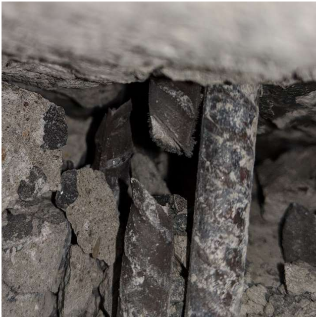
d) Rupture of vertical web reinforcement at wall base
