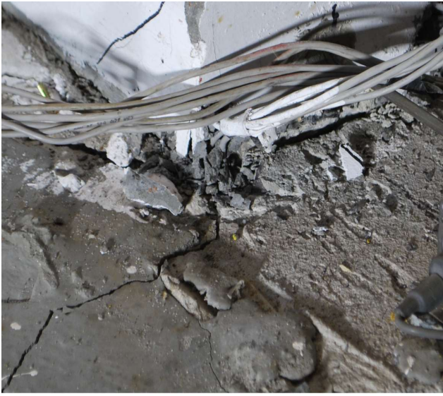
d) Cracks in the foundation at drift stage = 2.3% (East)
