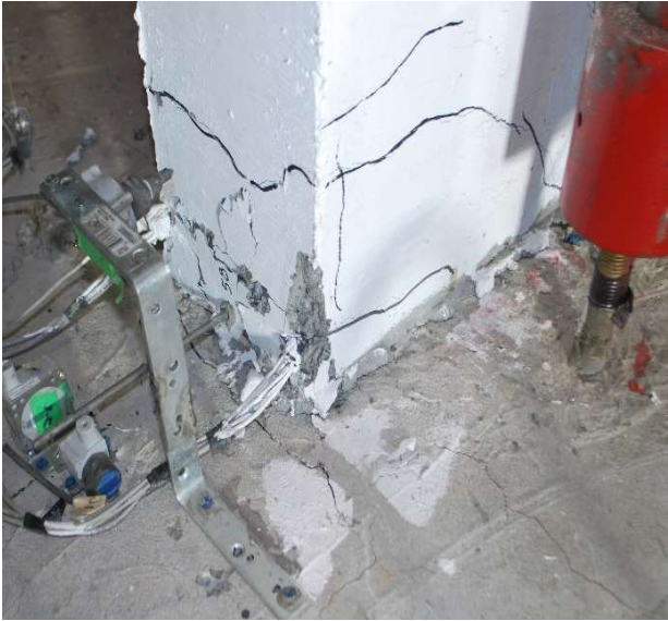
a) Cracks in the foundation at drift stage = 1.1% (West)
