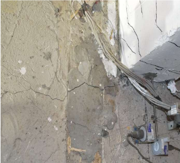
b) Cracks in the foundation at drift stage = 1.1% (East)
