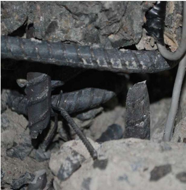
c) Rupture of boundary element longitudinal reinforcement at wall base
