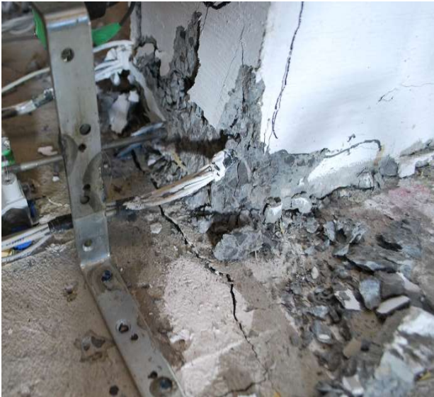
c) Cracks in the foundation at drift stage = 2.3% (West)
