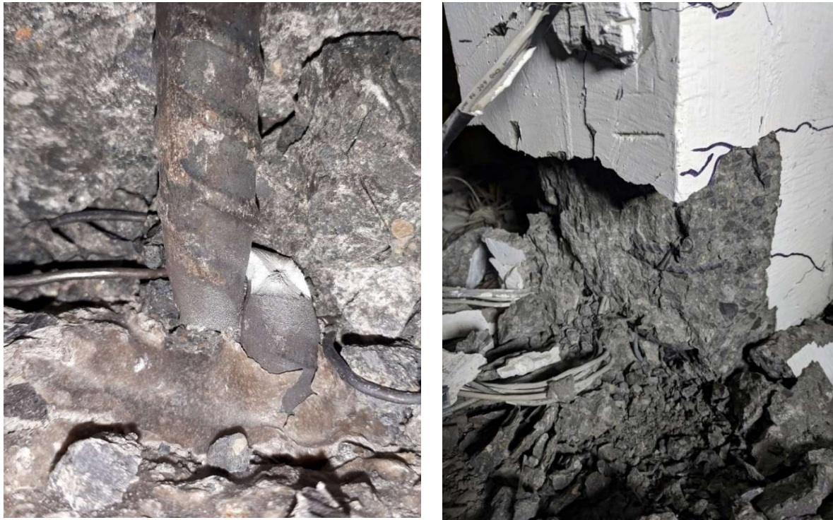
a) Ruptured longitudinal reinforcing bar in the west side boundary element
