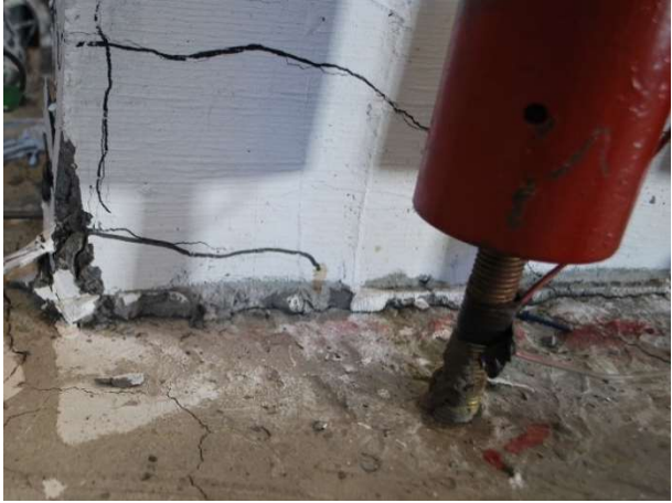
a) Crack at wall base at drift stage = 1.9%
