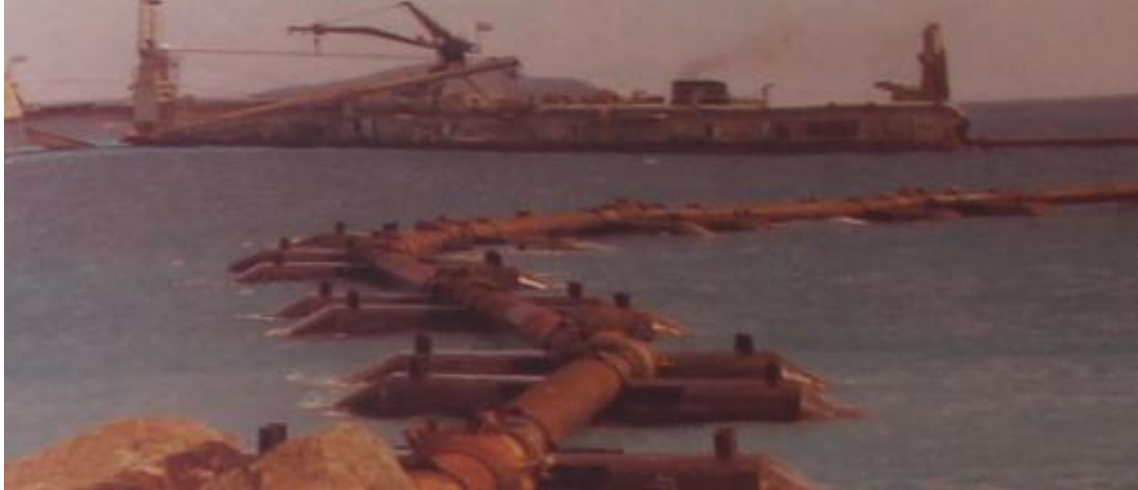
Figure 2.3: Dredging Activity in Jetty Bay during the Airport's Construction (Skylarc Pictures inc., 2015)
