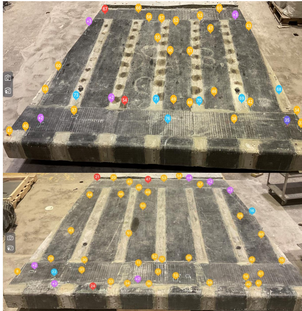
B.0.3- Defects on top surfaces of Diaphragm #3 side I (on the top) and side II (on the bottom)
