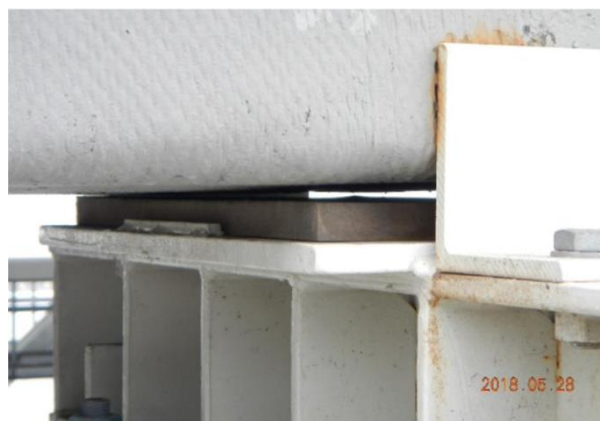
Figure 2.2 - Corrosion leading to discolouring of CFRP protective layer (4W-5W) (Stantec, 2018)
