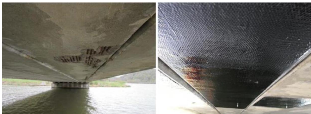
Figure 2.14 -Whiteday Creek Bridge a) before repair b) After CFRP repair (Joshi, 2018)
