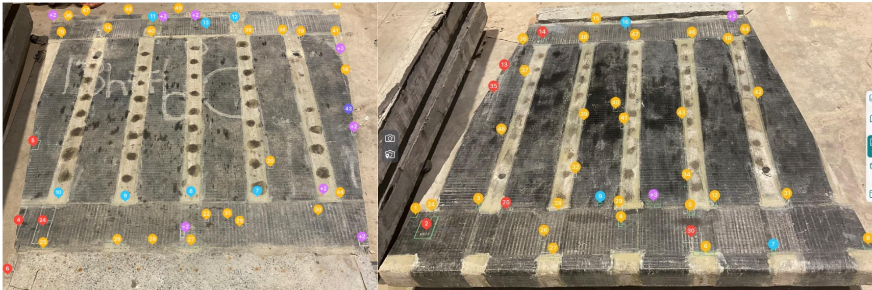
B.0.1 -Defects on top surfaces of Diaphragm #1 side I (on the left) and side II (on the right)
