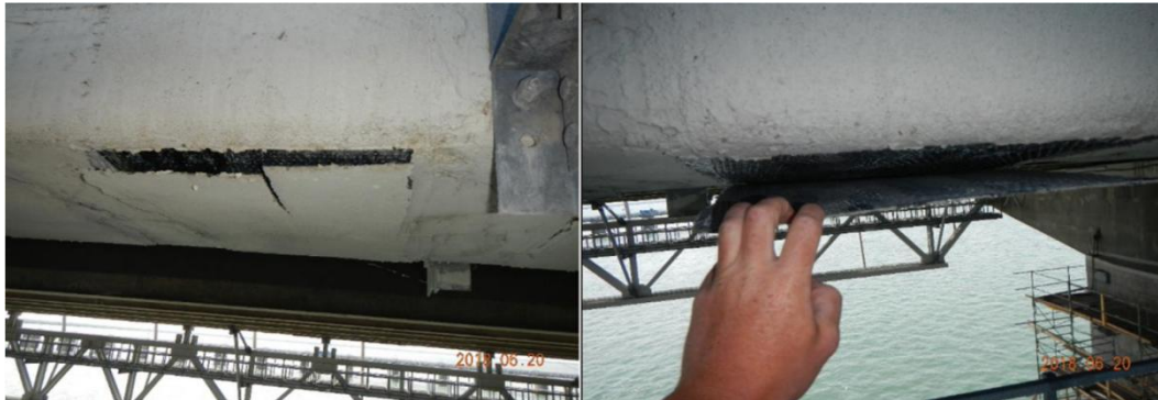
Figure 2.3 - Detachment of CFRP protective cover (Section 5; 22W-23W) (Stantec, 2018)
