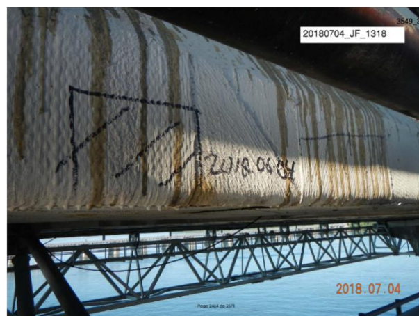
Figure 2.5 -Stained protective coat due to leakage (Stantec, 2018)
