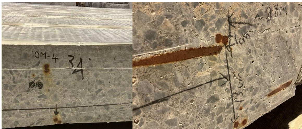
Figure 4.8 -Random placement of rebar without sufficient spacing or concrete cover a) side A of diaphragm #3 b) side B of diaphragm #3
