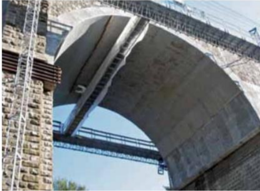
Figure 2-16: Strengthening an unreinforced concrete bridge in Italy with PBO-FRCM composite (ACI 549.4R-20).
