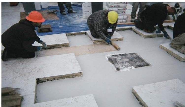
Figure 2-20: PBO-FRCM placement on the roof around the duct for strengthening (ACI 549.4R-20).
