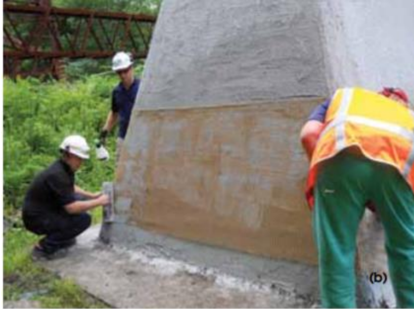
Figure 2-19: One sheet of PBO-FRCM composite is being applied to the surface (ACI 549.4R-20).
