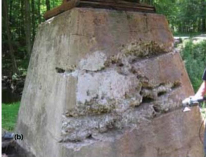
Figure 2-17: The deteriorated surface of a pedestal ( ACI 549.4R-20).
