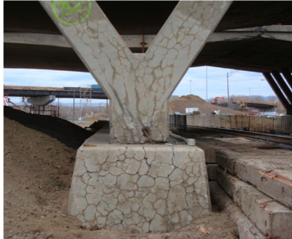
Figure 1.1: Map-cracking on the surface of AAR-damaged concrete [6].
