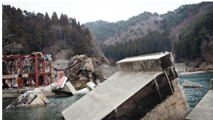
Figure 1.4 - Failed breakwater in Kamaishi, Japan [Sasaki, 2011]
