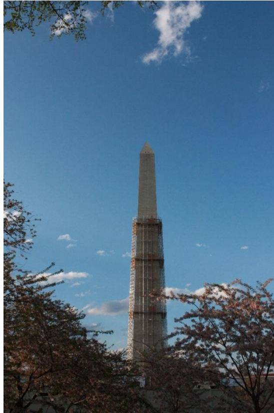
Figure 1.4. Restoration work in the spring of 2013 on the Washington Monument in Washington DC following the August 2011 M5.8 Virginia earthquake (Photograph: S.K. Ploeger).
