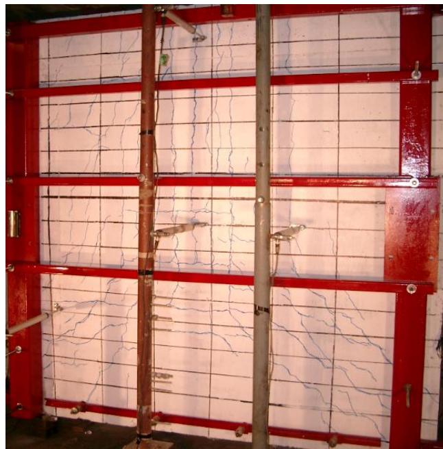
Figure 6.20: Condition of Wall 1 after test 5
