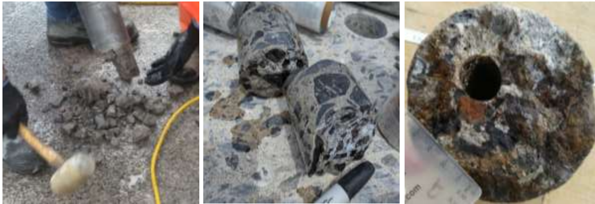
Figure A 9 Core specimens from the PS displaying damage
