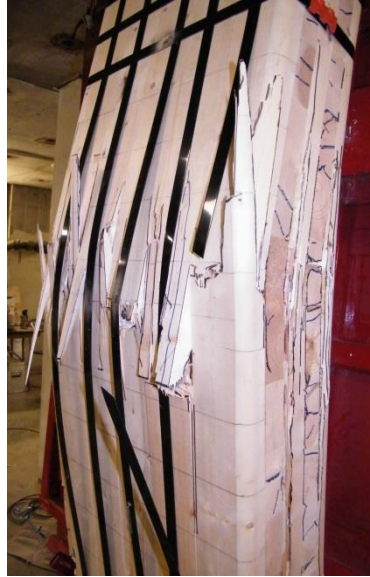
Figure 4.29: CLT5-3 Flexural Failure
