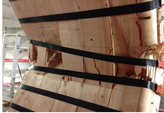
Figure 4.39: CLT5-D1 Compression Failure
