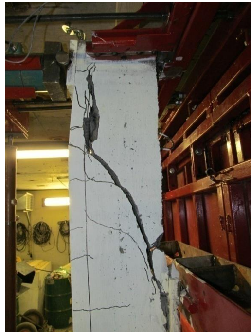
(b) Shear Failure of Blast 2
