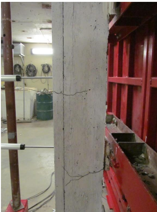
(a) Mid-Span Damage, Result of Blast 2
