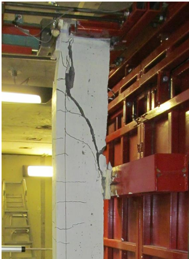
(a) SCC 0% Shear failure at Blast 2
