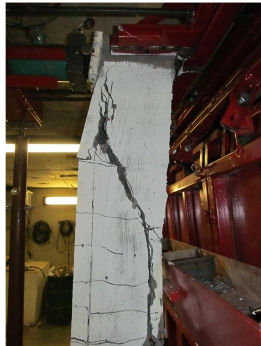
(b) Shear Failure of Blast 4
