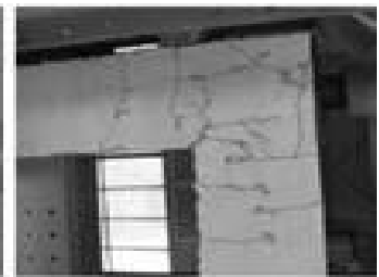
c) Cracks at ultimate disp.
