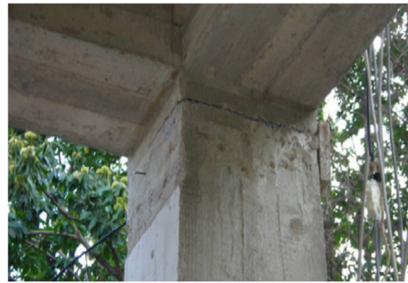
Cracking at beam-column joint: control building (1 st Storey)
