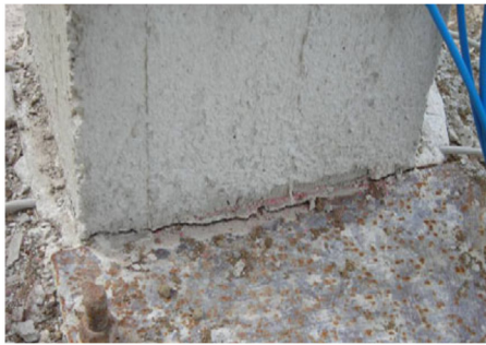
Reinforcement slip at column base: control building (1 st Storey)
