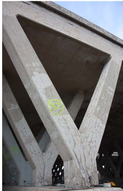
Figure 4-10. RBC exposed pier: a. FE overall damage (plastic strain) with original RH, b. FE reinforcement stress with original RH, c. FE overall damage (plastic strain) with global RH, d. FE reinforcement stress with global RH, e. FE overall damage (plastic strain) with local RH, f. FE reinforcement stress with local RH (stress values are in Pa), g. Overall observed damage.
